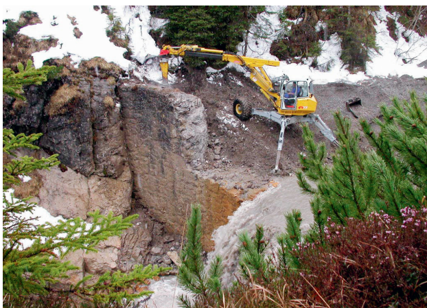
Figure 1: Dam removal at the Hornbach (Tyrol). To reduce river-bed degradation and related safety risks at the Lech River, several sediment control structures - up to 16 m high - were removed in relevant tributaries. At the Hornbach, 900.000 m 3 of bedload are released again step by step, contributing substantially to ecosystem functions and habitat availability. About 16 km of river-stretches are reconnected (Credit: Toni Vorauer/WWF).
